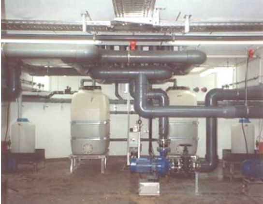
Underground pump station. Photo INTEC
